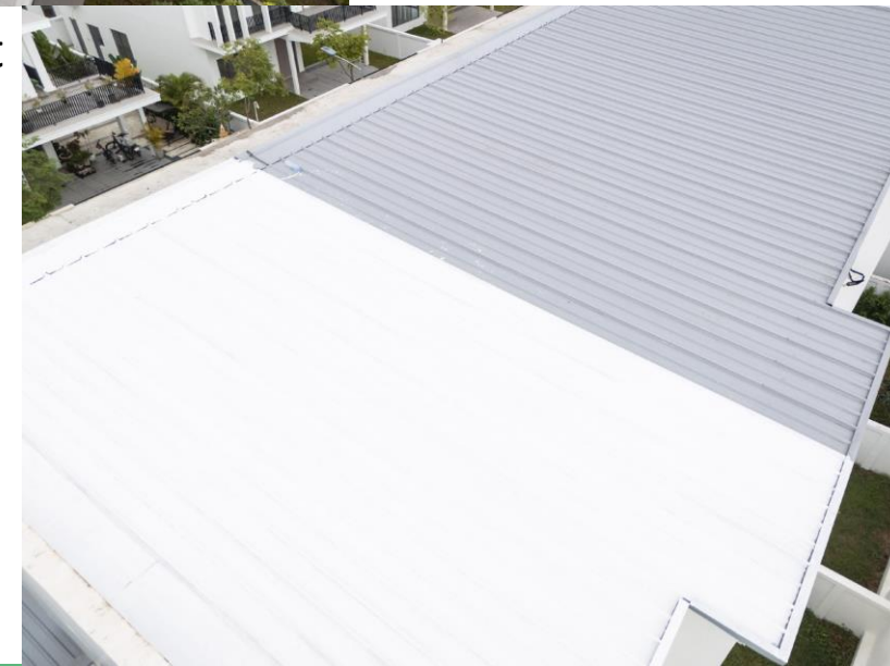
Cool Roof on PCS Integrated Unit
