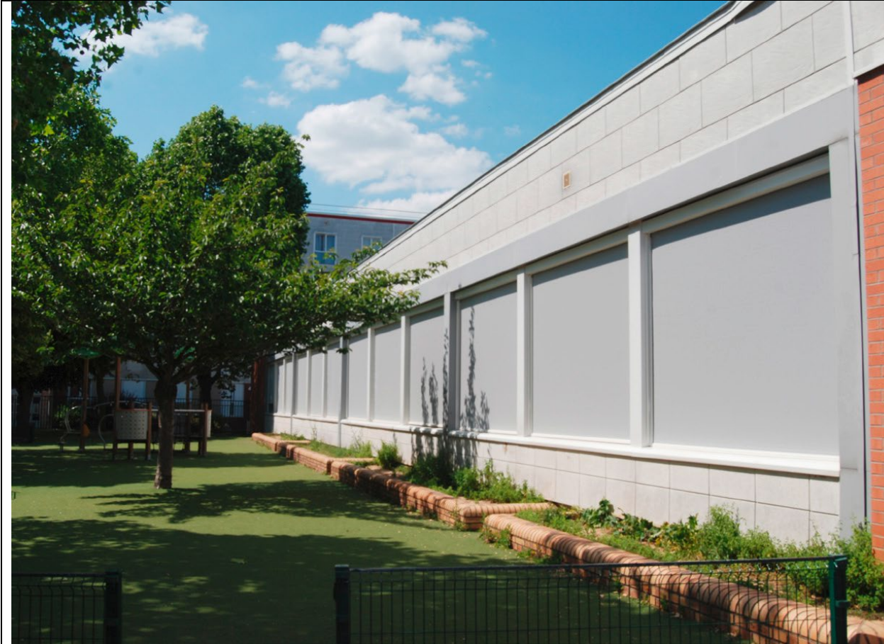
Outside view of the façade with exterior motorised ZIP blinds.
